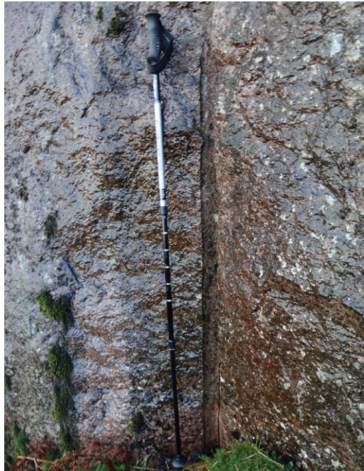
Photograph 3. Shot hole drilled in quarry face, made with triangular section. (A Wainwright)
