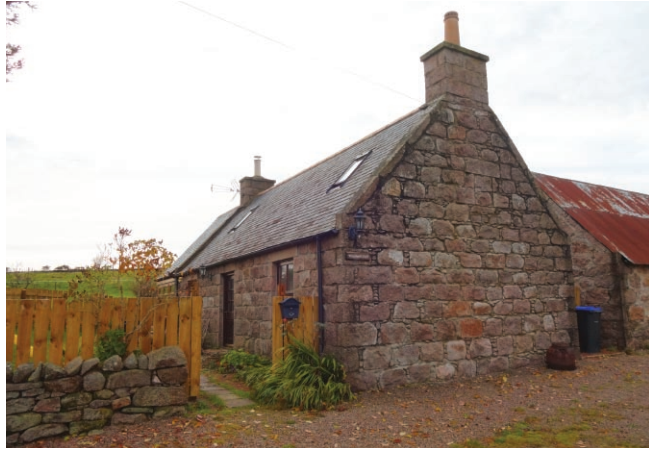
Photo 3. Burnside of Braco. Small four roomed cottage. Note the stones on the gable end, all with rounded corners. These are field stones that have been dressed to some degree. (Photo by the author)
